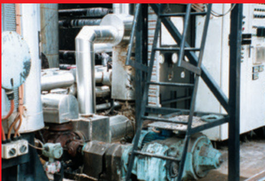
Fixed installation EBSRAY model G25 pump in Bitumen Blend Plant.
